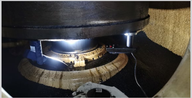
The stroke length and position of the piston is found by using laser.
