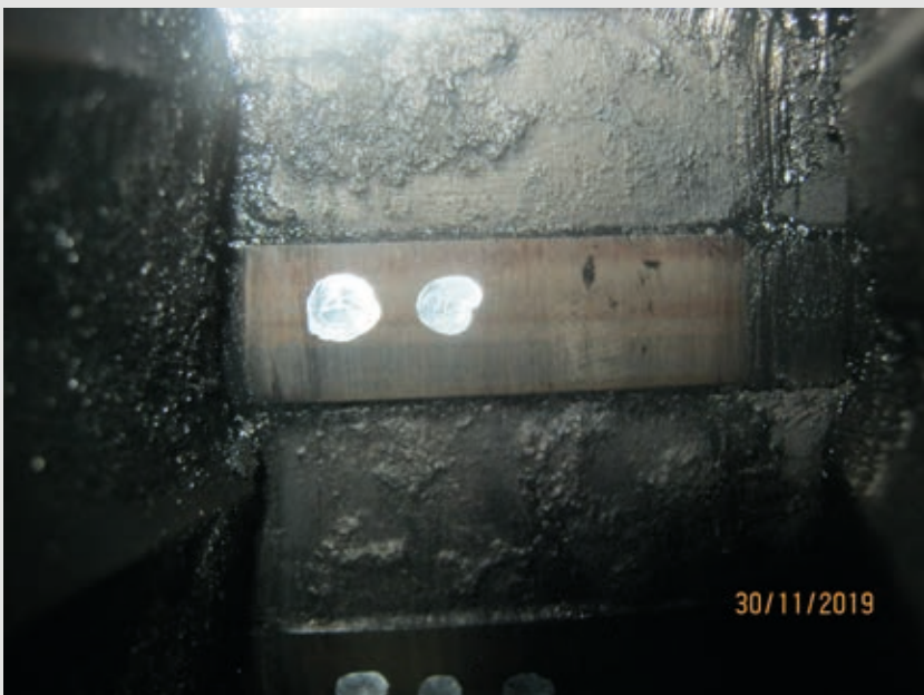
High degree of visible contamination on the piston rings.
